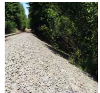
Tall fill slopes above Cedar Creek at MP-27.2.
