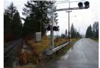
Most of the Chelatchie Rail crossings of roadways have warning signals similar to this one at NE 182nd Avenue.
