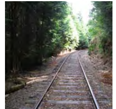
Steep slopes on both sides of the corridor near MP-30.2.
