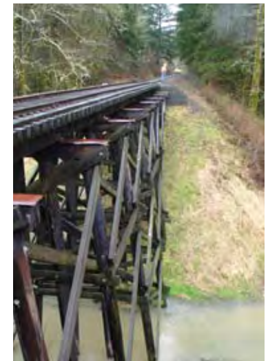
The design and condition of the existing Chelatchie Prairie Railroad bridges make them unsuitable for adding trail uses in combination with active rail operations. Bridge 18 south of Heisson.
